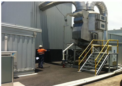
Air-conditioning systems installed by NDMS
