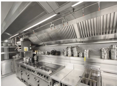
Complicated network of ventilation systems
